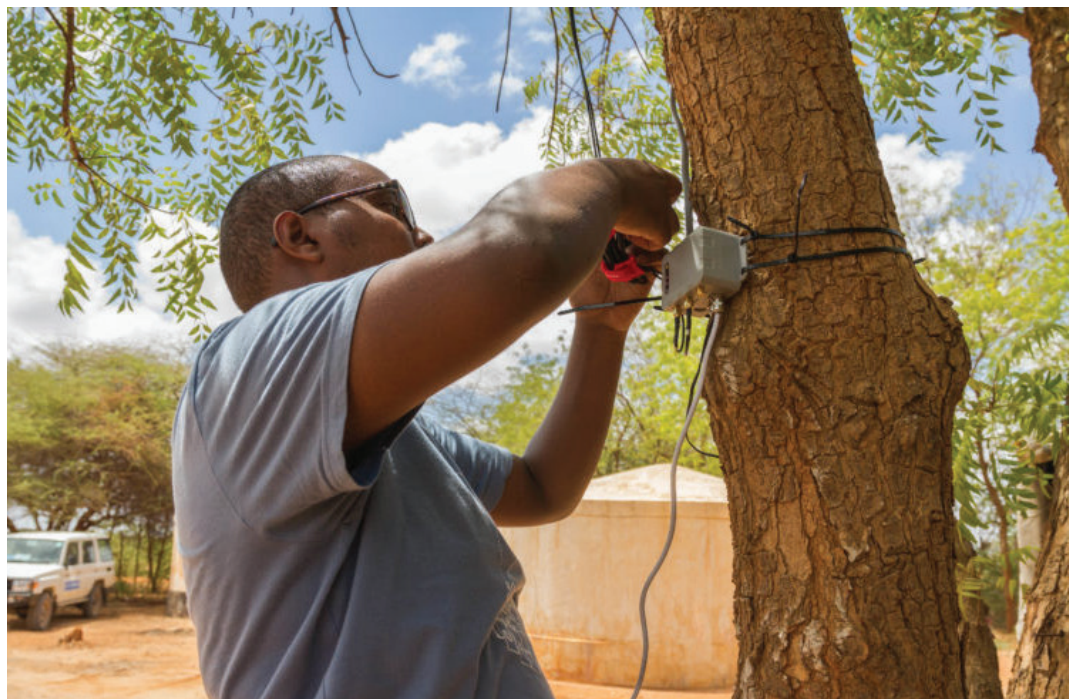
BRCK, UNHCR project instalation source: https://www.brck.com/about/blog/
